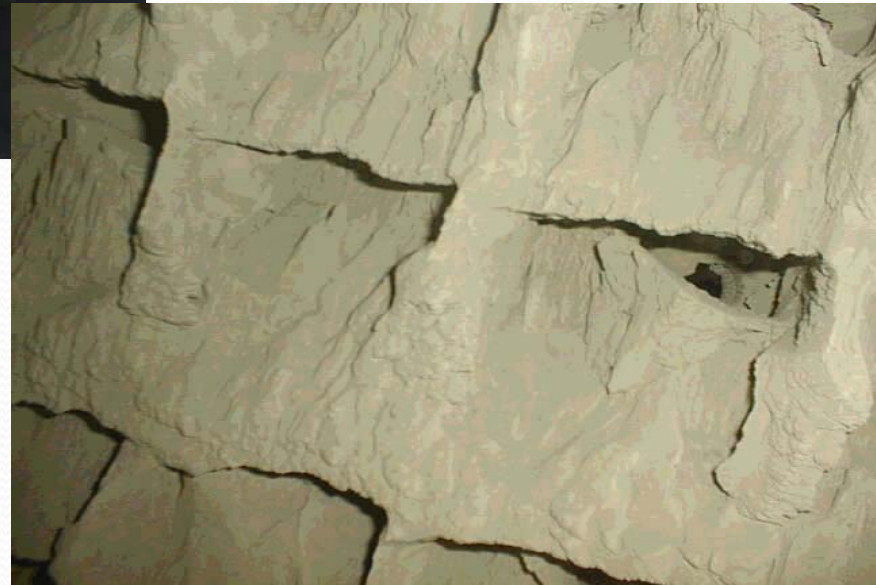
Air Preheater Fouling
